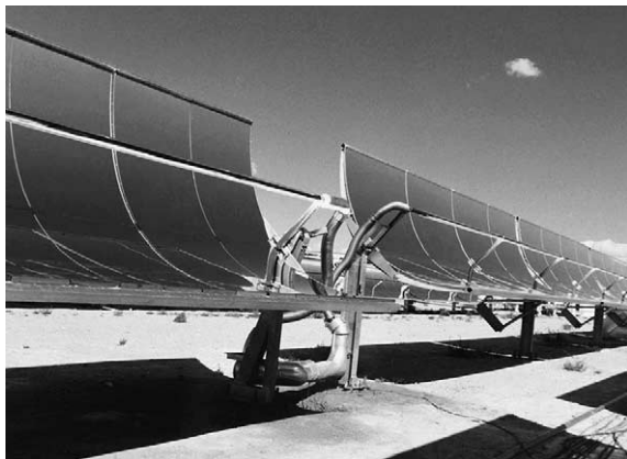
Fig. 1. A portion of an LS-3 plant at Kramer Junction, California.
