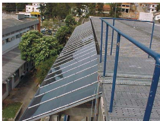
Figure 1: View of the 2kWp grid-connected, building-integrated, double-junction a-Si PV system installed at LABSOLAR's building in Florianopolis – Brazil (27°S).
