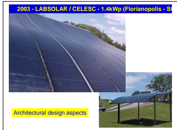
Fig.6: Florianopolis – SC; one of the three BIPV systems installed in a joint project with the local electricity utility CELESC to monitor the performance and showcase grid-connected PV. All three installations are fully monitored, to accumulate experience in the operation performance of grid-connected PV systems.
